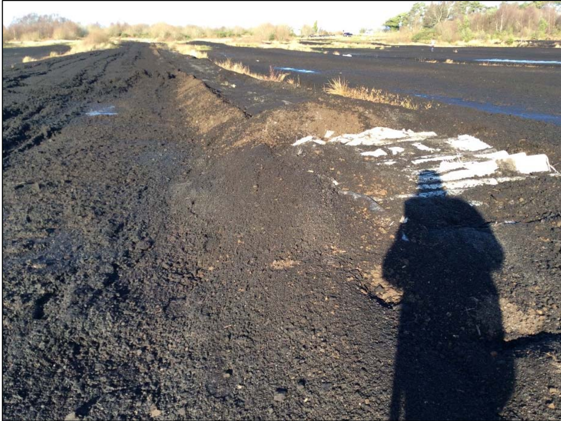
Plate 13.5: Site of OF030-063 Class 3 Togher in location of decommissioned railway looking north.
